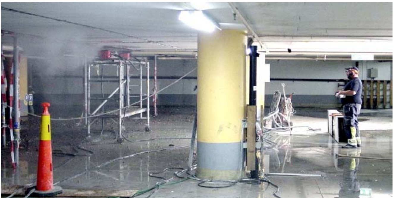
Conjet Jetframe 101 NALTA mounted on standard rolling scaffolding exposing joints in the ceiling of a parking garage. The operator monitors and controls the process at a safe distance from the working area.
